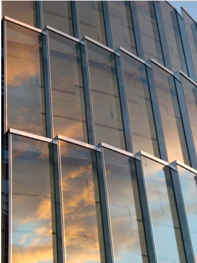
Serrated, inclined structurally glazed twin skin with perforated bronze anodised sheeting behind.
